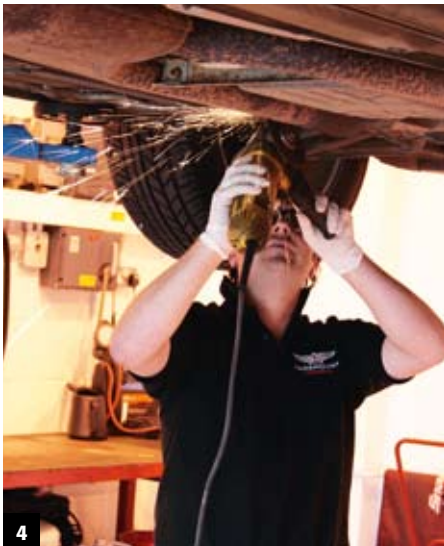
4 Given that the old system was going in the bin, Paramount didn't waste any time and simply cut through the seized retaining fixings. The pipes were also cut into sections to make removal easier
